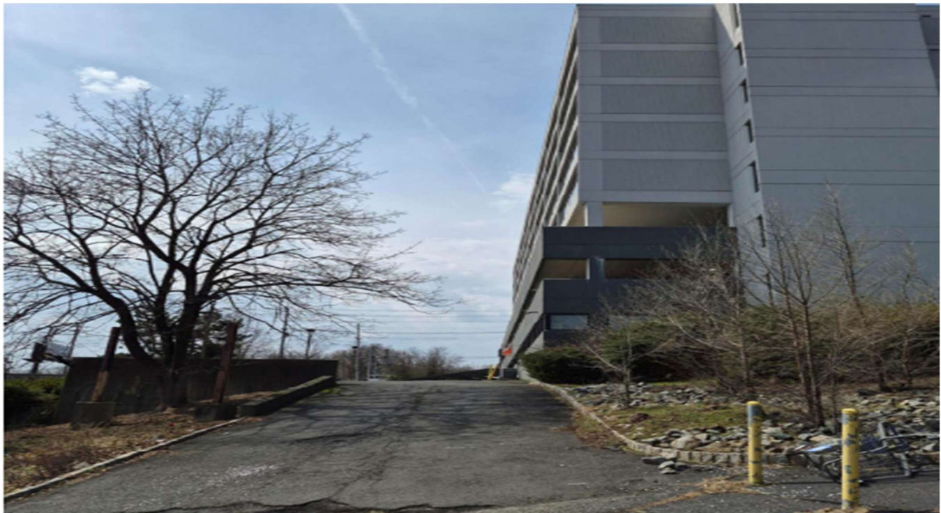
Photo 2: West view along the driveway and circulation area adjacent to the hotel building, showing pavement condition and building-site relationship.
