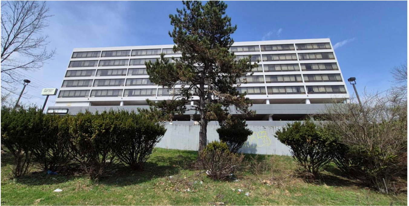
Photo 1: East view of the hotel building and frontage landscaping, showing the dated exterior condition and site frontage context.
